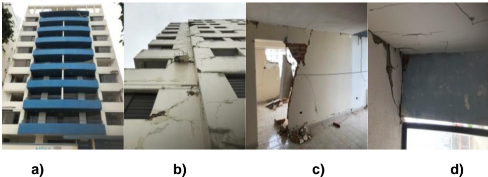
Figure 12. (a) The Spondylus Building of 9 floors of reinforced concrete; (b) Building's facade, major damage of masonry is not observed.; (c) Collapsed masonry supported by an electrical duct; (d) Cracking in relieved slab on facade window.
